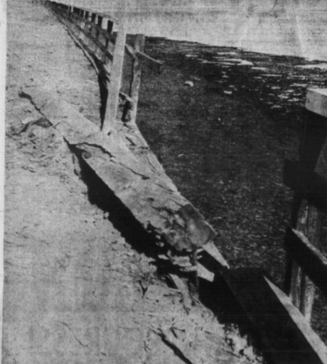
THE DILAPIDATED appearance of the structure is shown here. Much damage was the result of a recent heavy rain storm which was accompanied by higher than normal tides. It was recently suggested by Mayor A. Wallace Gaudet that Prime Minister Diefenbaker be shown the condition of the breastwork on his visit to the province today in an effort to obtain federal aid for repairs. However, G. R. Foster, president of the Progressive Conservative Association said this
