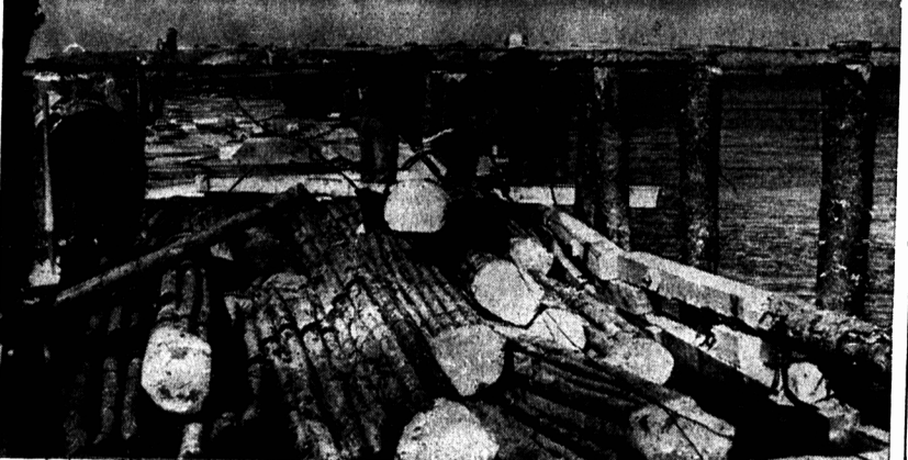
When the composite rolls have been dumped, workmen with crow-bars and peaveys work in conjunction with the truck and towing cable to inch them into place between the piles in the channel.
