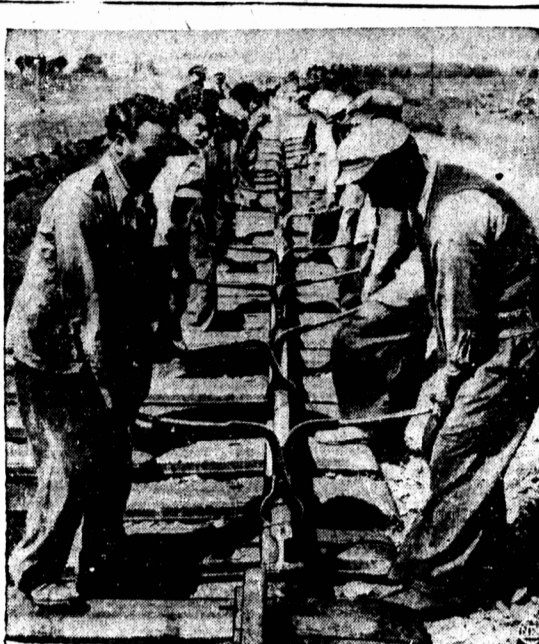
GREECE SNAPS BACK —With hand tools and plenty of elbow grease, workers at Salonika, Greece, put a newly-arrived steel rail into place to repair one of their many war-damaged lines. A full consignment of rails shipped from Western Europe was unloaded and set into place in one day, dramatizing the return to pre-war efficiency of Greek railroads.
