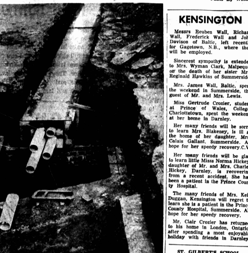
ENCLOSED IN A cement castra constructed in a shallow trench a few inches beneath the cement surface of Water Street, are the pipes which will carry all communication lines underground on Water Street in Summerside between the two railway crossings. On top of the cement casing a single heavy lead cable will be laid which will supply electricity to street lights in this area. The pipes, which are seen above, lead into a large brick-lined manhole in front of the telephone office where servicing and maintenance work can be done. The communications lines will be located in these pipes, and will eliminate all overhead lines and poles, with the exception of street lighting stanchions from the main Summerside business area.
