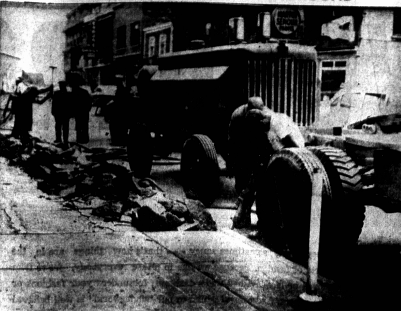
WITH THE AID of power drills, workmen are busy tearing up the outer section of the sidewalk along the south of Water Street in Summerside where underground communication and street lighting cables will be placed between the railway crossings on the east and west ends of Water Street. This will eliminate all communication and power lines and poles in this area which will have sixteen steel stanchions for street lighting, and five manholes to service communication cable junctions. After the installations are completed the wide sidewalks in the vicinity of Holmans and Smallmans Stores will be about 30 inches narrower, allowing this additional area to be used by motor traffic in this busy business area.
