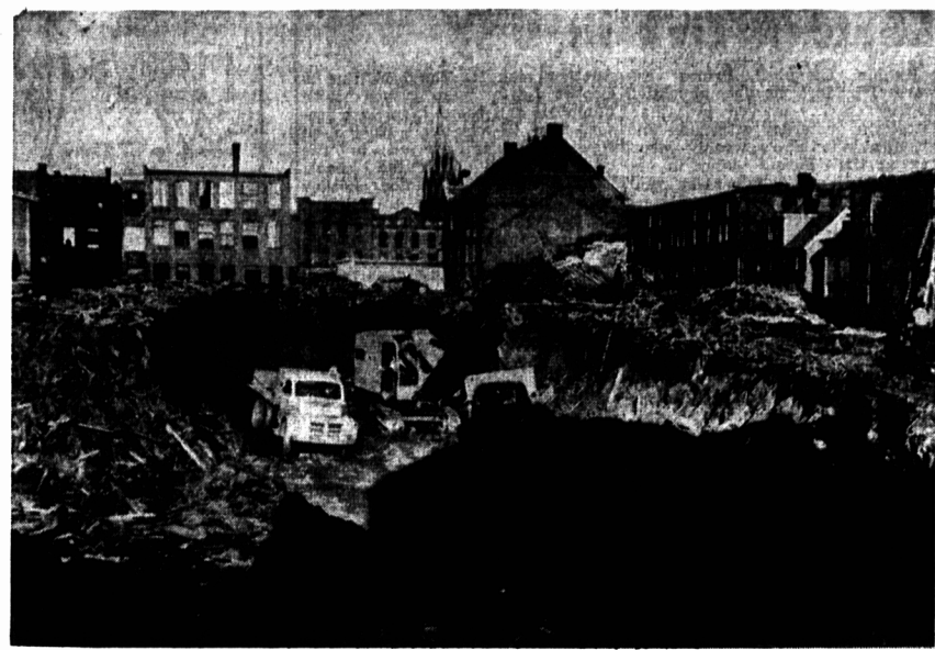
Only last Monday houses lined the Richmond and Sydney Street sides of the Federal Building Block. Today little remains but broken laths. The power shovel eats its way through the length of the every 2 1/2 minutes. (Photo by Margaret Mallett).
