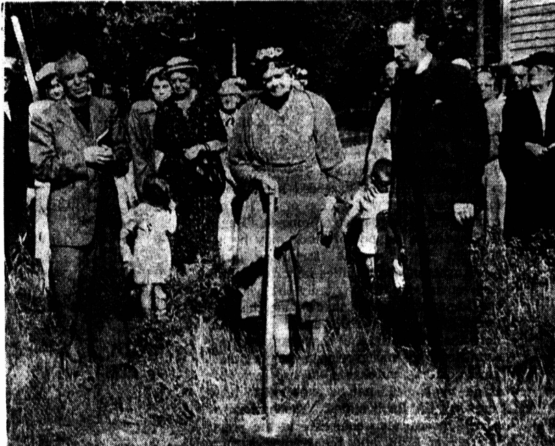
Turning the first sod on the site of the new Church of Scotland building on Birchwood Street on June 25. The ceremony was conducted by Rev. J. H. Bishop, Minister of the Church of Scotland (left), assisted by Rev. Allasdair Johnston (right) representing the Free Church of Scotland. The first sod was turned by Mrs. Maria Mutlow, (centre) who, bordering on her 90th year, is the oldest member of the congregation. —Barter's Film Lab.
