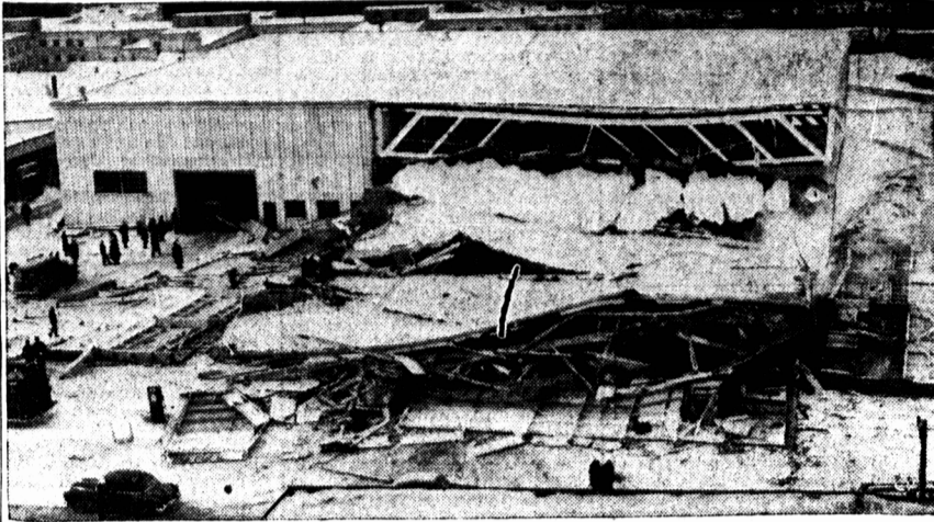
$320,000 GARAGE COLLAPSES—The new $320,000 motor-transport and administration building at Shearwater naval air base across the harbor from Halifax, considered an armed forces showpiece, collapsed mysteriously. Naval officers said they believe the building may be a total loss. There were no injuries. Government agencies have retained an outside expert to investigate the collapse of the newly-built garage.—(CP Photo).
