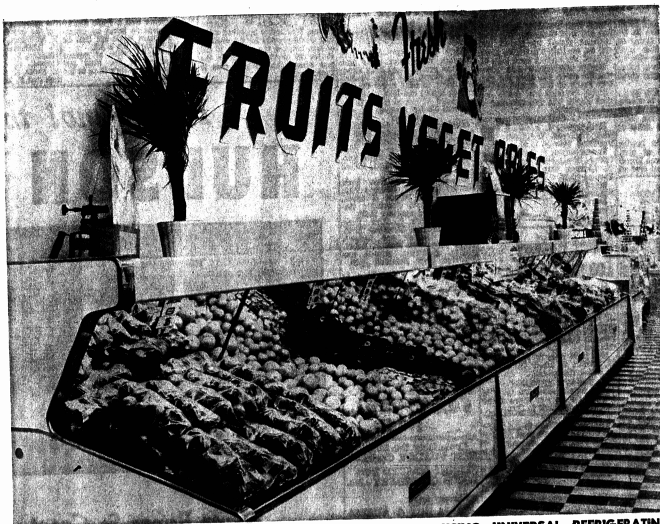
THIS IS A TYLER FRUIT DEPT. — INSTALLED BY PALMER ELECTRIC — USING UNIVERSAL REFRIGERATING EQUIPMENT
