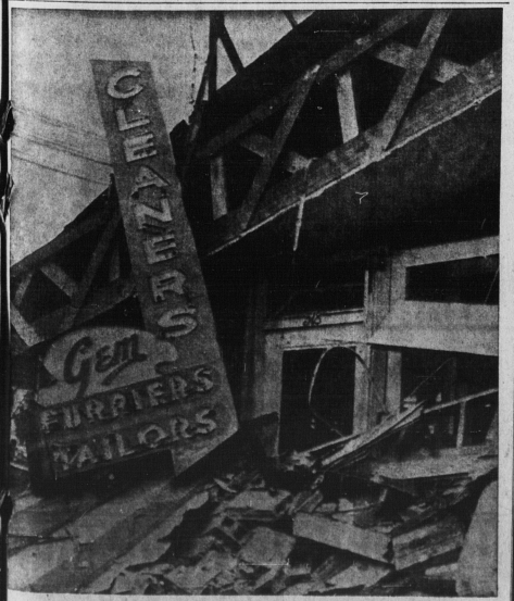
10 ESCAPE IN BUILDING COLLAPSE Ten occupants of this Ketchikan, B.C., cleaning establishment escaped as the front wall fell into a lot where excavation is underway. The 10 were evacuated from the building by an RCMP staff sergeant who happened to be passing as the structure collapsed. (CP Wirephoto)
