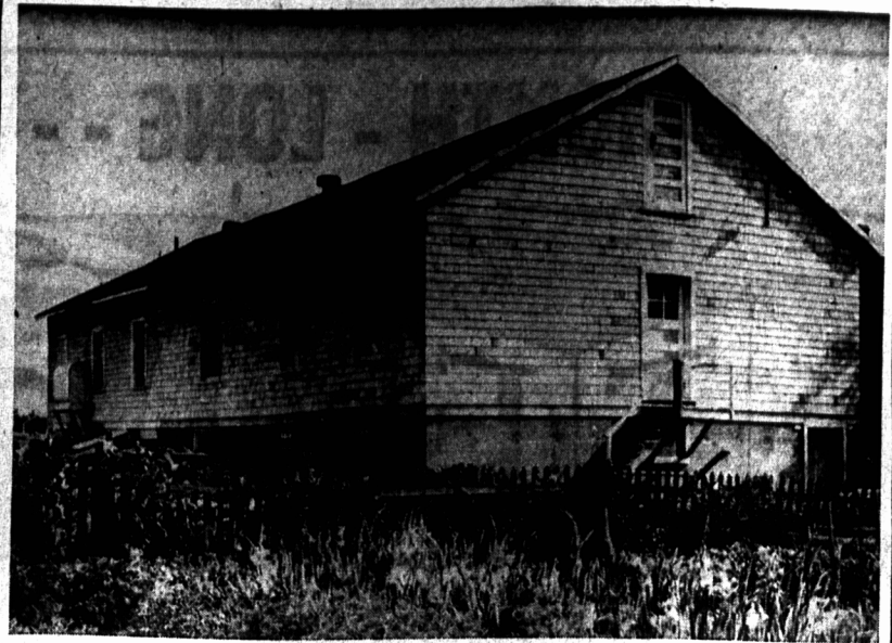
EXTENSION TO S'IDE Y CENTRE A rear view of the Summerside Y Center shows the results of a forty-foot extension, almost completed, which provides the Y's Men with a building 60 by 31 feet. The main floor contains an office, kitchen and an auditorium measuring 66 by 31 feet. The main floor provides accommodation for the Y's Men's Club, the Y's Menettes Club, three H Y Clubs and a Phlat Club, while the full cement basement will be used in continuing the work of Boy Scouts, Wolf Cubs and Brownie groups in Y's Men's Club. The Y's Men's Club has a membership of 51 men and about 49 ladies belong to the Y's Menettes Club. The renovations to the building will cost approximately $4500 and the building committee composed of James Connell (chairman) Keith Pickard, Laurie Coles, Jack Scott and Ben Champion. The work on the building extension is being done by Gerald MacLean of Kensington as carpenter foreman and he is assisted by three other carpenters. The Y center is situated on the south side of Green Street between Streets opposite the ball diamond at Queen Elizabeth Park.
