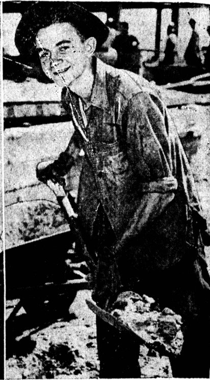
second summer as a trust company clerk. Attacking earth with shovel and plenty of enthusiasm is Ron Owston, 17, a construction laborer who says: "I like it."
