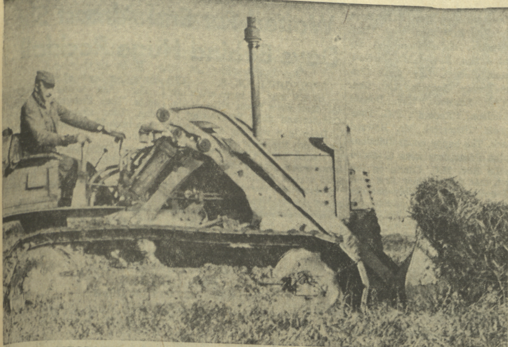
WITH A BULLDOZER commencing its first work on the site of Hillcrest Park in preparation for the construction of the first
