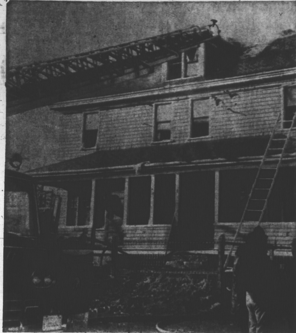
CITY DWELLING DAMAGED BY FIRE
