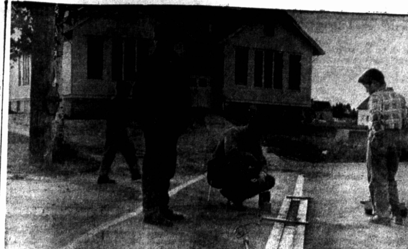
Cross walks being sprayed on the Montague Memorial School by Mr. Gilbert Clements, of the Junior Board of Trade, in front of their use. The project is being sponsored by the Junior Board of Trade, in front of their use. The project is being sponsored by the Junior Board of Trade, in front of their use.
