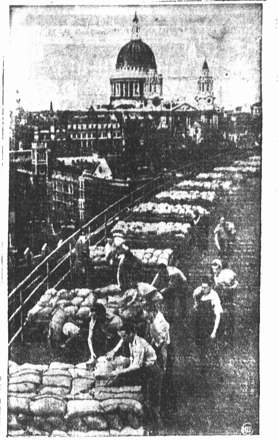
Working furiously against time, these workers pile layers of sandbags atop a London office building as protection from high-explosive bombs that would rain on the city as soon as war started. Unprotected and a shining target, is the stately dome of St. Paul's Cathedral in the background.
