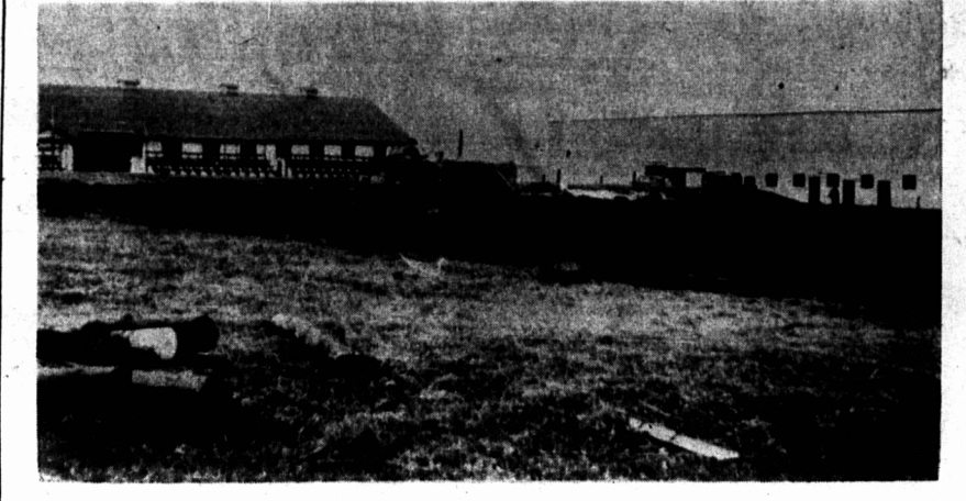
A County Construction Co. bulldozer levels the ground on which the new Agricultural Exhibition Building will be erected at the Provincial Exhibition grounds. Barter's Film Lab.
