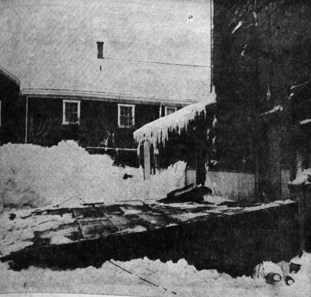
A ROOF, which provided protection for drive-in patrons of the Island during Tuesday night's severe storm, collapsed yesterday morning from the weight of the heavy snow which blanketed the western end of Summerside.
