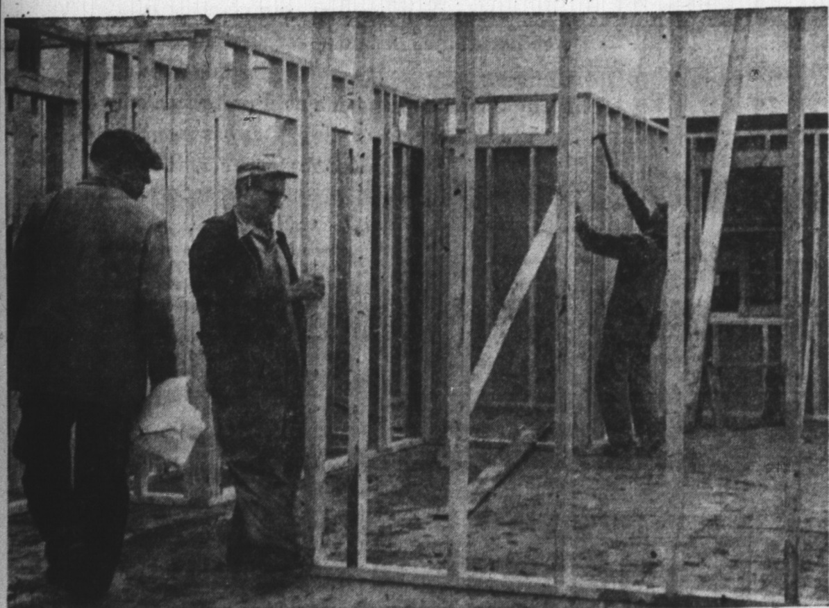
8:45 a.m. The pre-engineered factory built exterior walls sheathed with HOMASOTE were completely erected by 8:10 a.m. This photo taken at 8:45 a.m. shows the erection of the interior partitions which were completed by 10:00 a.m. under the guidance of our supervisor.
