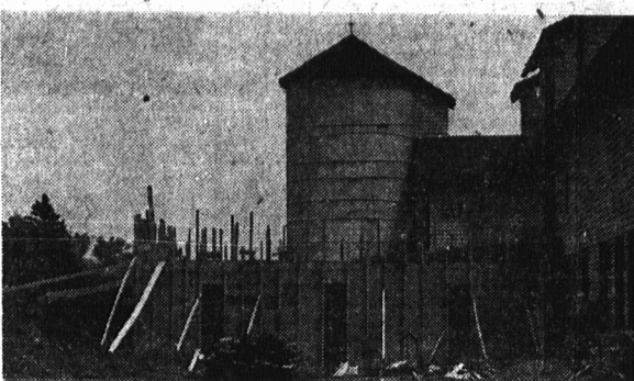
Shown in the above photograph is a trench silo for grass silage in the process of construction at the local Experimental Station.
