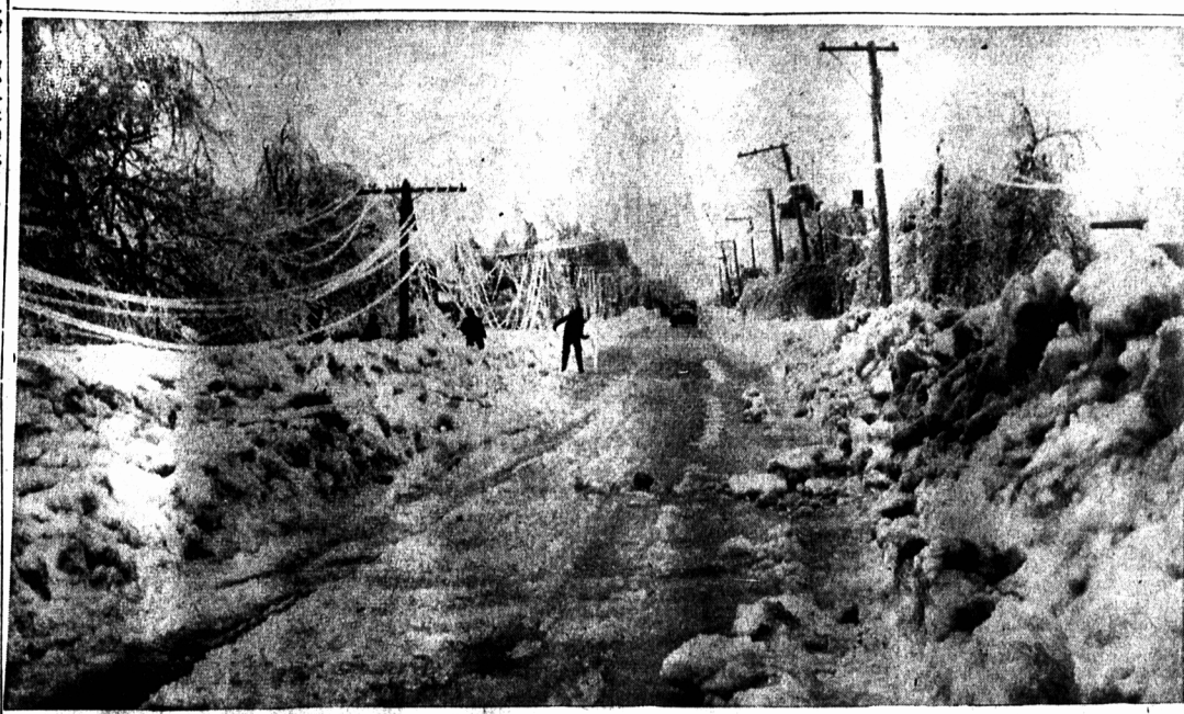
WORKMEN CLEARING the tangled mess of telephone and power lines from a street in Tignish following the weekend ice storm. Conditions similar to this and worse exist throughout the whole Prince County area. Hard work is gradually improving conditions.
