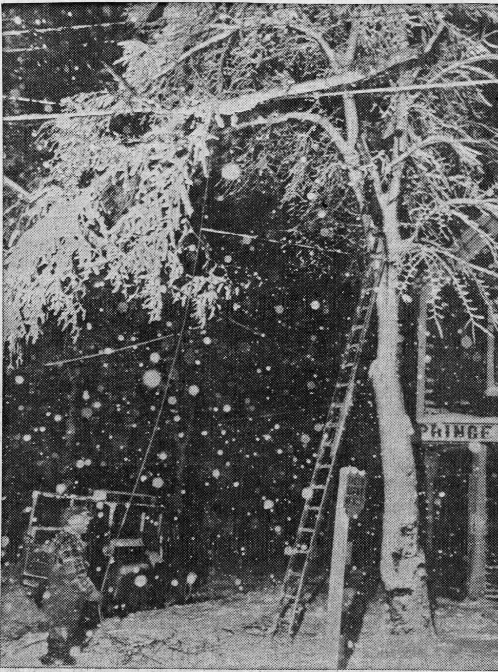
LINEMEN Carl Moore (left) and Reuben O'Hanley (in the tree) remove a branch threatening one of the city power lines. Work was performed around 9:00 at the height of last night's sleet p.m., at the corner of Prince and Water Streets.
