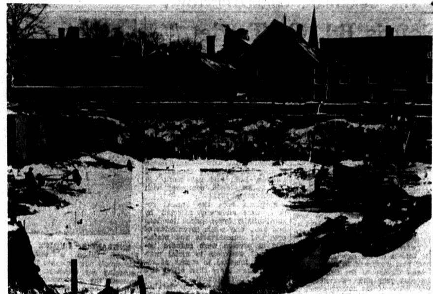
HOLE IN THE GROUND — Excavation at the site of the Eaton Store on Kent Street. —Photo by Barter
