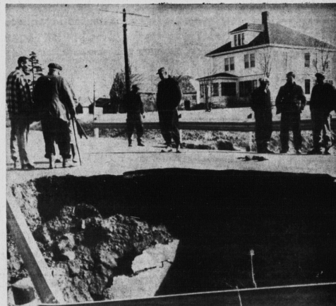
HOLE IN BRIDGE AT MONTAGUE
