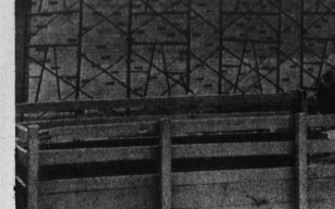
Increasing the elementary classrooms space in St. Elizabeth's is being constructed by Robert Rankin Construction.
