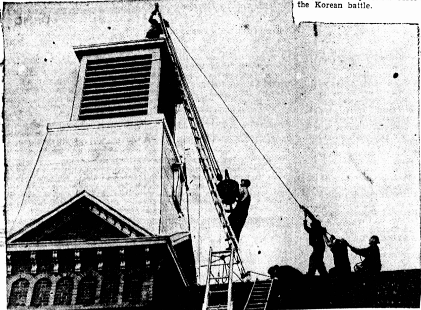
Johnston Murray directs movement of the 300-pound siren. Cline Bagnell guides it up the ladder. Reminiscent of last war preparations in Canadian towns was the placing of a combined air raid and fire siren atop Orangeville, Ont., fire hall.
