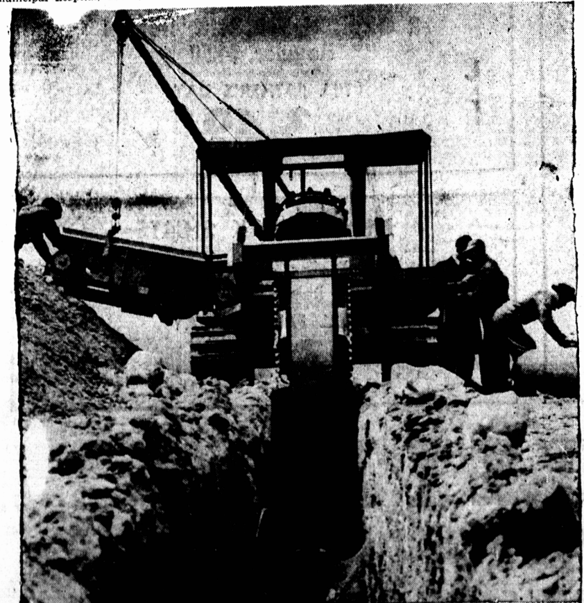
The building of $90,000,000 Inter-provincial oil pipelines from Edmonton to Superior, Wisconsin, is a job for big machines. Here, one of largest trenching machines ever to operate in Canada, is seen digging out a five-foot ditch, which would ordinarily take 500 men to complete. The 1,150-mile pipeline, which is expected to be completed by fall, will be used to market Alberta oil to U.S.
