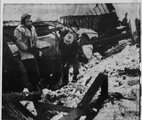
COLD TASK It was sub-zero as crew members worked yesterday to repair the Canadian National
