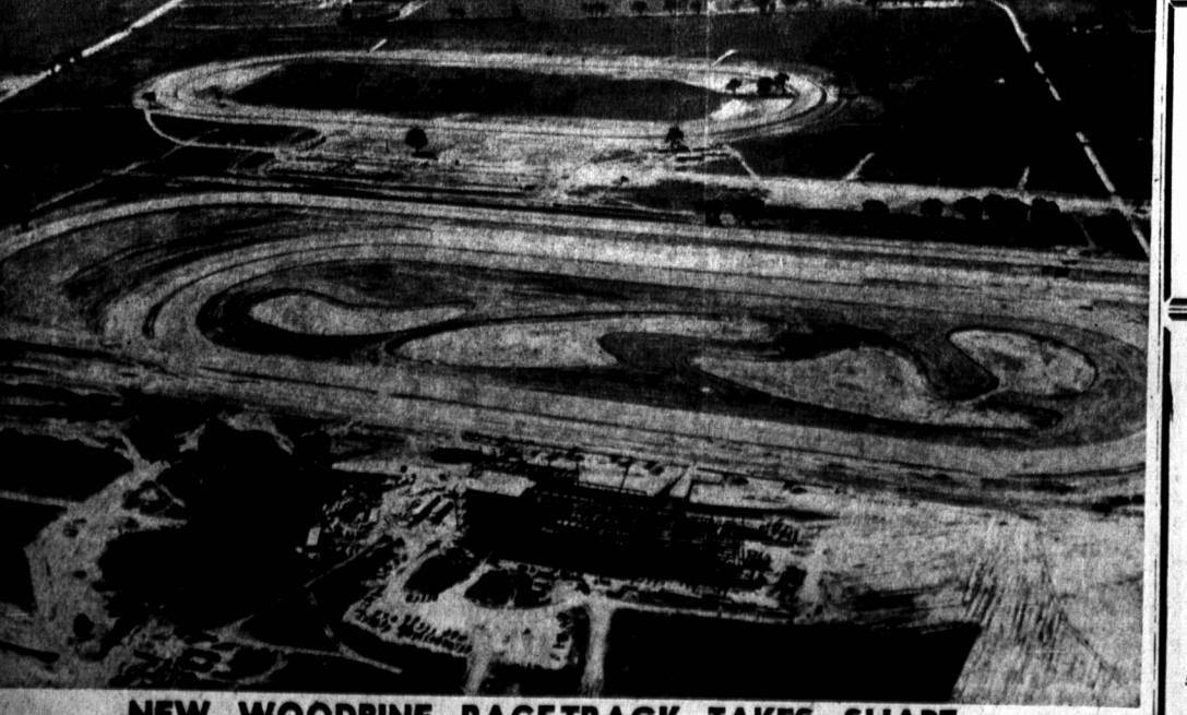
NEW WOODBINE RACETRACK TAKES SHAPE Construction takes shape on the new $10,000,000 Woodbine race track which will open in the Toronto suburb of Malton next fall. The new layout, to be the richest race course in Canada, covers an 800-acre property, and replaces the 70-year-old Woodbine in east-end Toronto. This aerial view shows the four tracks in background and construction of grandstand (centre) which will seat 8,000 persons to start. (CP Photo)
