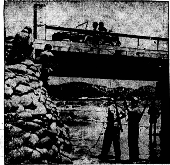
MEN AT WORK —As a 1st Cavalry Division jeep rolls across this bridge near Yongdong, Army engineers prepare to blow up the span. They're connecting wires to detonate charges placed under the bridge. Other GI's stand watch. (Photo by NEA staff correspondent Ed Hoffman.)
