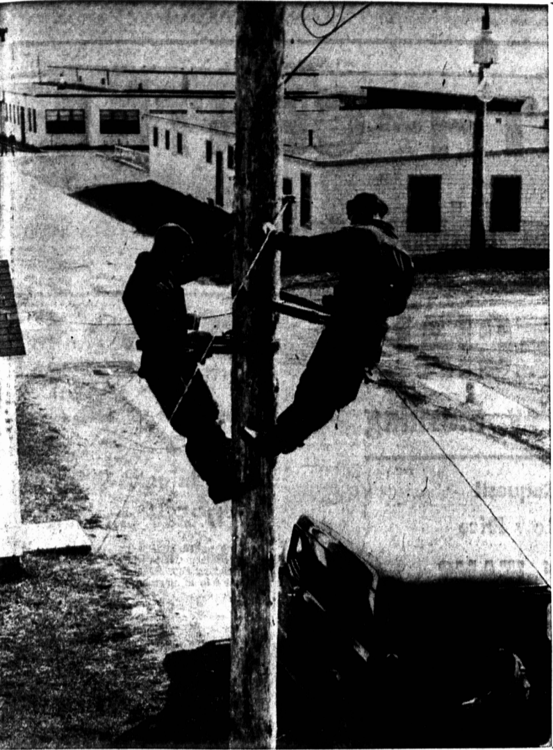
INSTALL COMMUNICATION lines. - Members of East Coast Signal Regiment of Halifax are in Summerside this holiday weekend installing permanent communication lines throughout the RCAF Station. Working with regular RCAF personnel, the militia regiment has been replacing temporary communication lines with ones of a more permanent nature. Above, Sergeants Bud Backman and Ken Luddington work high above one of the base's many streets.
