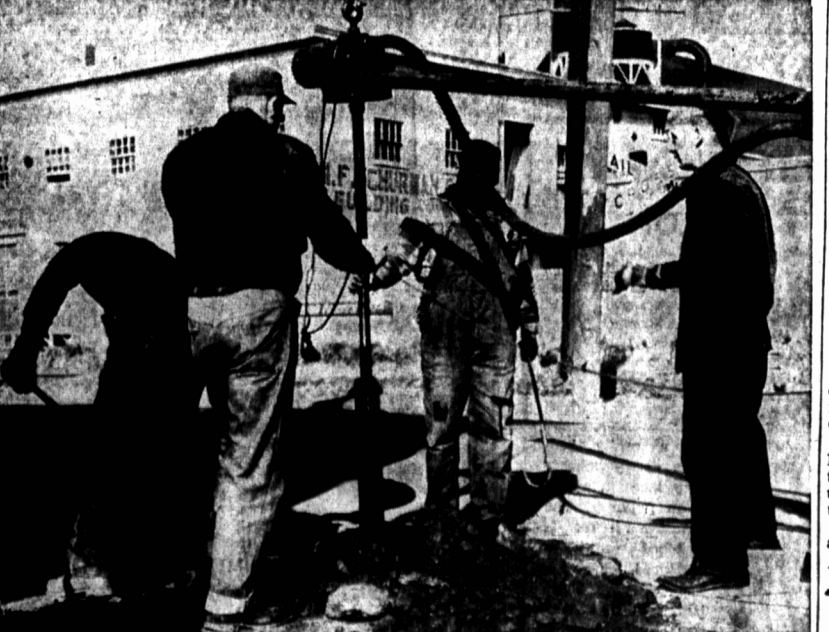
Beginning the excavation for the eastern terminal of the underground communication system being installed between the east and west railway crossings in Summerside, workmen are seen yesterday just east of the M.F. Schurman Co. plant as they begin operations with a rotary drill in preparation for completing the eastern
