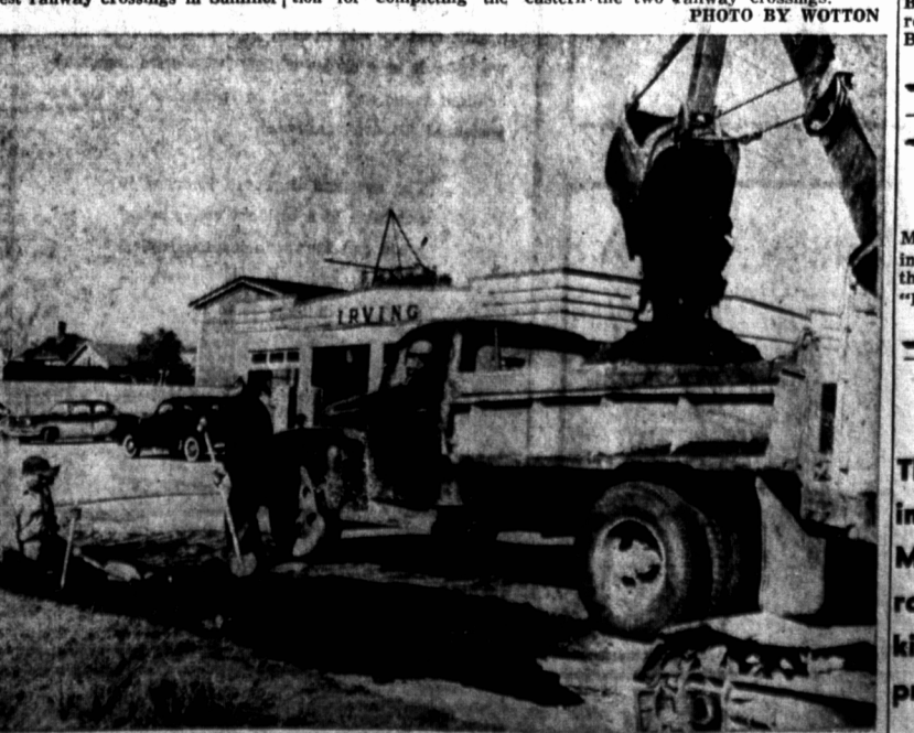
Excavating a trench in which the communication and street lighting cables will be placed underground between the two railway crossings on Water Street in Summerside, a big power shovel is seen yesterday loading a truck at the eastern crossing as work on the project nears completion. PHOTO BY WOTTON
