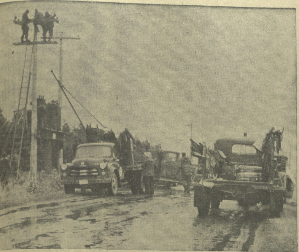
MARITIME ELECTRIC line remove the old sub station at Alberry Plains following the completion of a new sub station located near Summersville. The high voltage transmission line went into service Sunday and is now operating on 12,000 volts as an express feeder to serve Montague, Murray River and surrounding districts. Following the arrival and installation of transformer equipment at the Charlottetown sub station the line voltage will be increased to 34,500 volts.
