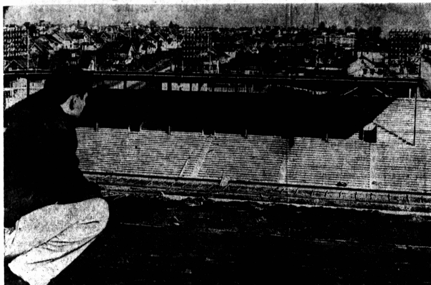
A workman surveys the new British Empire Games Stadium in Vancouver. This is an early construction shot of the $1,200,000 stadium built at Exhibition Park. After the Games it will be the home of B. C. Lions, newest entry in the Western Interprovincial Football Union, and will be known as Exhibition Bowl.—(CP Photo).
