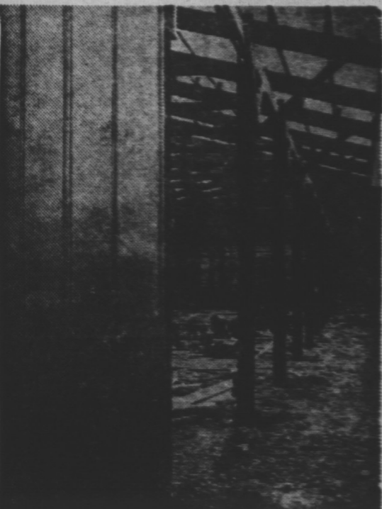
NO FOUNDATION IS NECESSARY for this low-cost steel building. Pressure-treated poles are set, framing members added and the galvanized roofing and siding nailed on.
