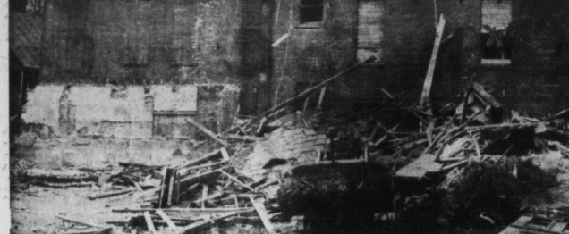
CH-TOWN LANDMARK BEING DEMOLISHED One of Charlottetown's historic old buildings, the former YMCA building on Richmond Street, is gradually being demolished by workmen in order to make way for a new recreation centre. The old building was one of the first buildings built exclusively for the use of YMCA members in North America. Two other buildings have also been demolished to make way for the new recreation centre. They were the old Aylward building and the Holy Name Hall. The Holy Name Hall was formerly the Zion Presbyterian Church and was built between 1857 and 1860.
