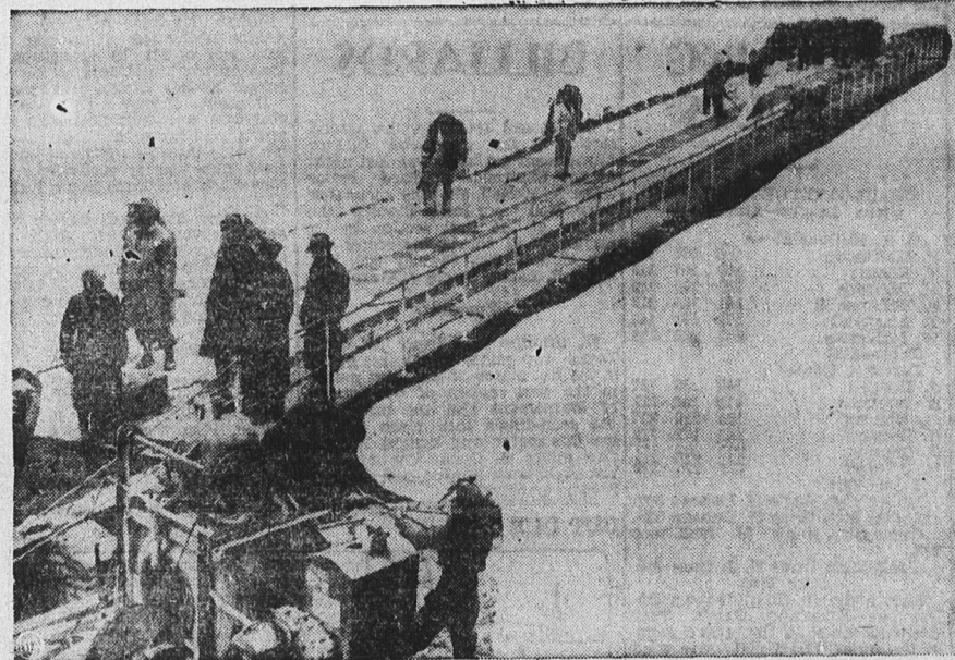
The structure pictured above is a long, temporary bridge constructed by Royal Engineers over a huge bomb crater in London. British censor didn't want to divulge its location, so had entire tell-tale background painted out before releasing photo for publication.
