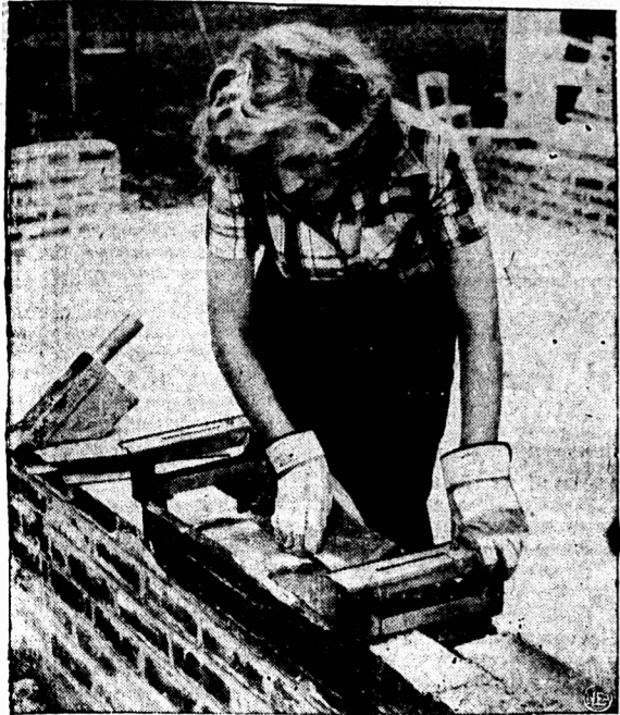
BRICKLAYING MADE EASY —The "first real improvement in five centuries in the method of laying bricks" is demonstrated in Montgomery, Ala., by coed Kitty McGlynn. The device, invented by engineers Paul H. Sommers and John S. Hodgson, is said to speed bricklaying four times the normal pace. Acceptance by the building industry could mean great savings in construction costs — especially in the building of low-cost homes.
