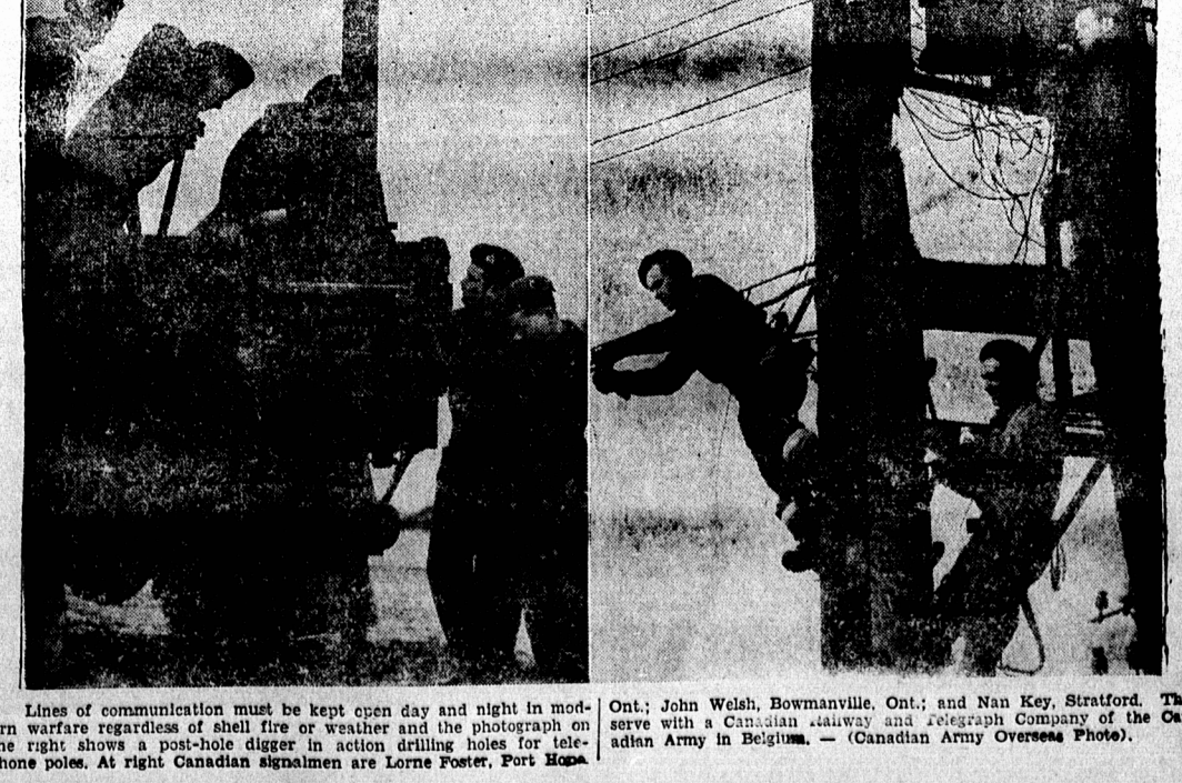
Lines of communication must be kept open day and night in modern warfare regardless of shell fire or weather and the photograph on the right shows a post-hole digger in action drilling holes for telephone poles. At right Canadian signalmen are Lorne Foster, Fort Hope.
