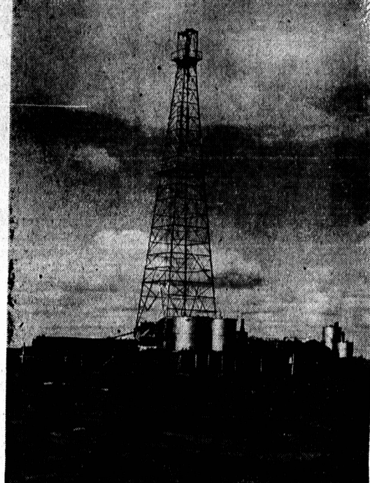
This is the 146-foot steel derrick on its man-made island in Hillsboro Bay on which oil drilling operations are underway.
