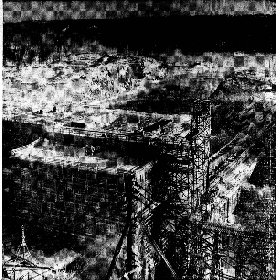
The dynamite used for blasting this huge rock cut would provide enough block-busters to blow Berlin to bits. This view shows tail race leading into the first half of powerhouse. It will develop power while second being built. Cold mist rising from water is result of 50-below temperature when picture taken.
