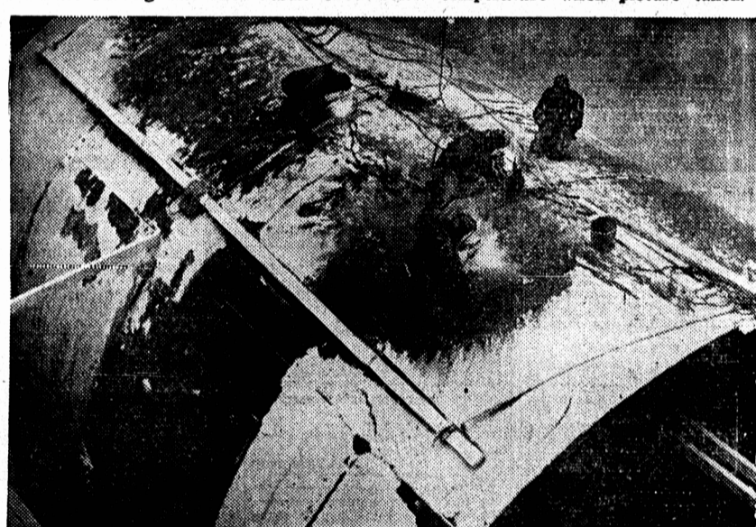
Welders crawl like ants on the belly of a section of the huge casing which lines concrete tunnels. Each tunnel is 30 feet in diameter, drops 200 feet, then runs 600 feet. Project will use 1,500,000 cu. yds. of cement.
