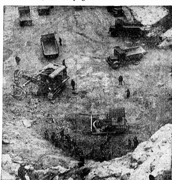
Forty-four power shovels and cranes, 525 trucks and 67 tractors are at present being used on excavation work to remove 7,300,000 cu. yards of rock and earth.
