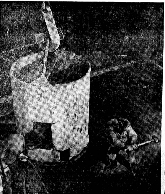
Ankle deep in concrete, workmen hang at huge bucket used for pouring cement mixture into forms for casing of "serole case" which will carry water to one of turbines.
