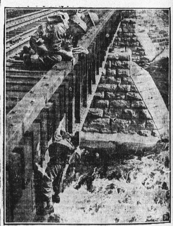
Demolition Squad. Glombering along a railway bridge high over a rushing torrent, this demolition squad is making preparations to "blow up" the structure during exercises at Petawawa training camp.
